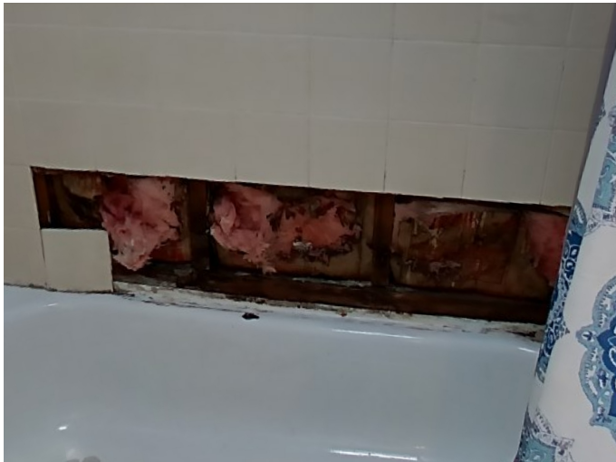
Condition: Holes in tub/shower surround
